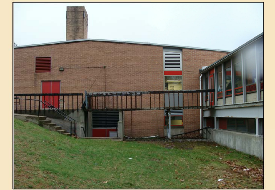
BELOW GRADE EXIT UNDER CONDEMNED BRIDGE
